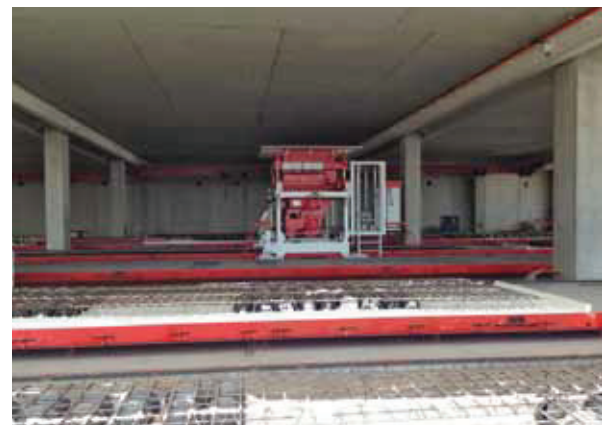
A view into the new Danstek factory building; Weckenmann supplied a production line of several hundred meters in length, complete with state-of-the-art equipment and machinery
