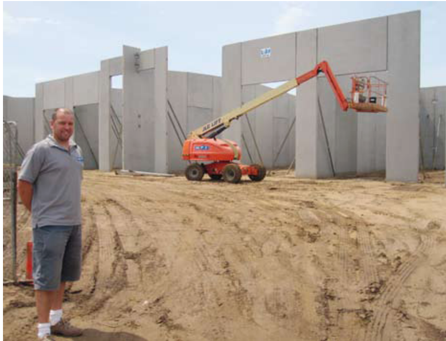
Fig. 4 Derek Finocchiaro on a construction site with precast concrete elements from MPC.
