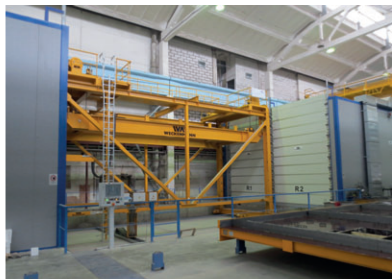
Curing chamber with hot air heating
